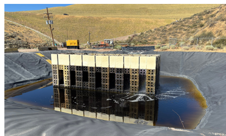
An EcoVap pilot evaporation tower at the Rain Mine North Waste Rock Disposal Facility.
